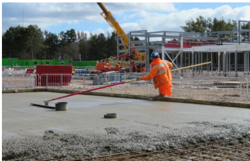
(Photo-'Marking a million hours': Contractor Oliver Payne floats the concrete to give a great finish on the foundation of a new Senior Ranks' Single Living Accommodation, Larkhill.)
